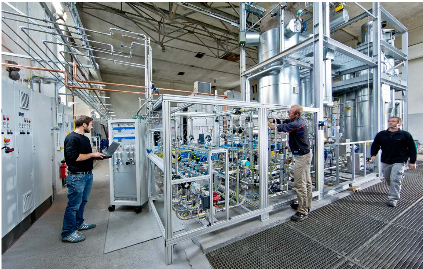
Power-to-Gas pilot plant at the Centre for Solar Energy and Hydrogen Research (ZSW), Baden-Wuerttemberg.
