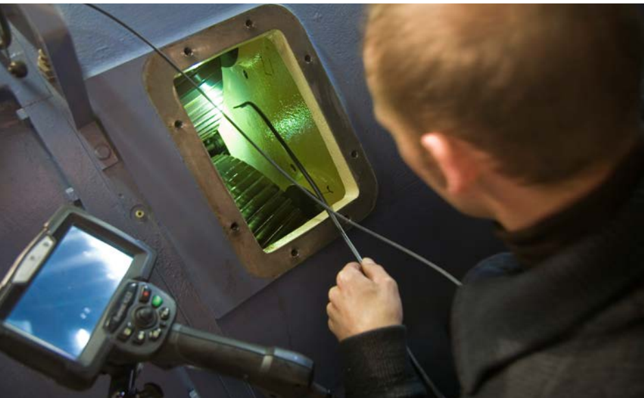
Video endoscopy to inspect the gearbox of a Repower MM82 at Drohndorf wind farm.
