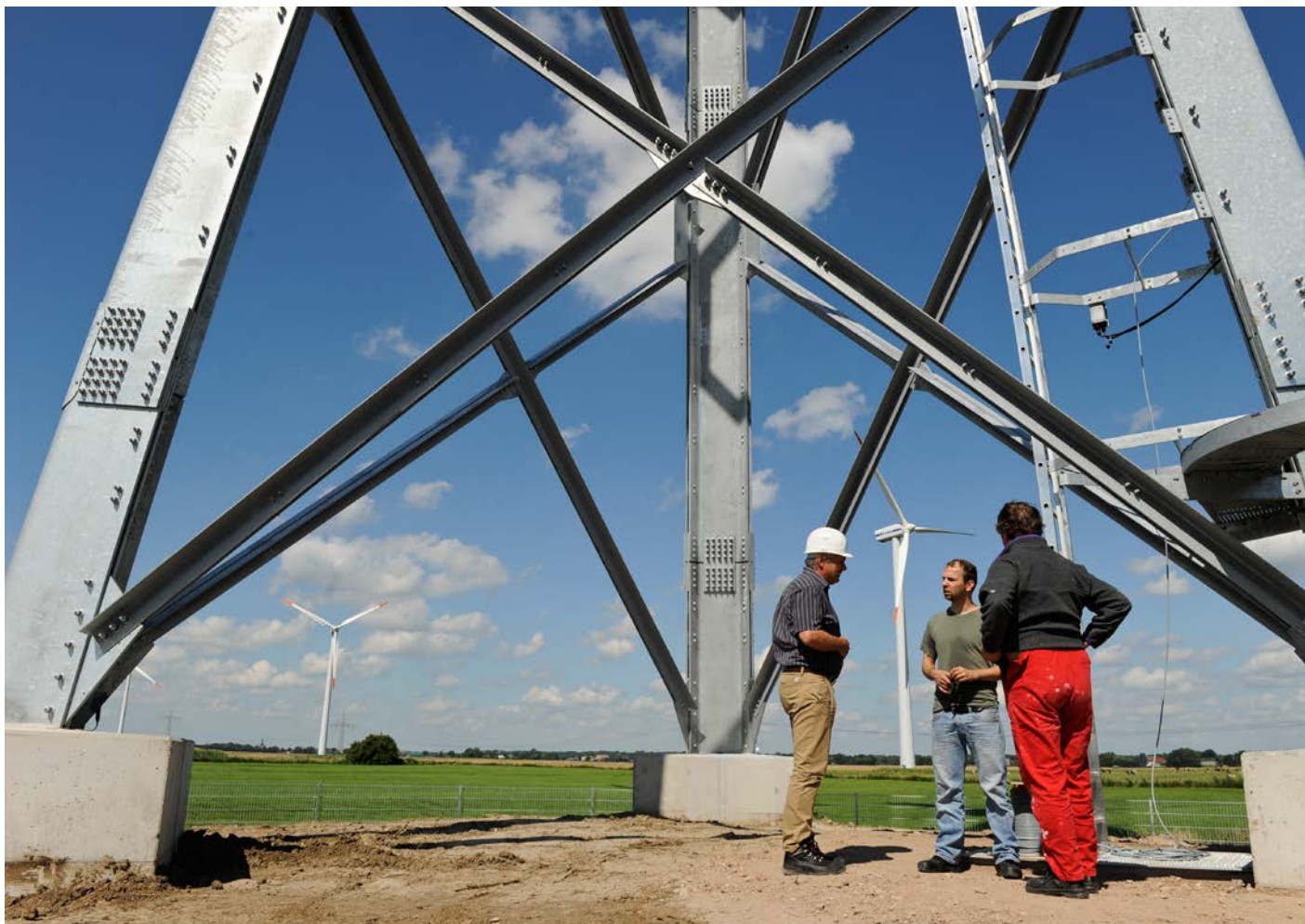
Onshore tripod: Erection of a new lattice steel mast construction for a Vensys wind turbine in Steinburg near Glückstadt.
