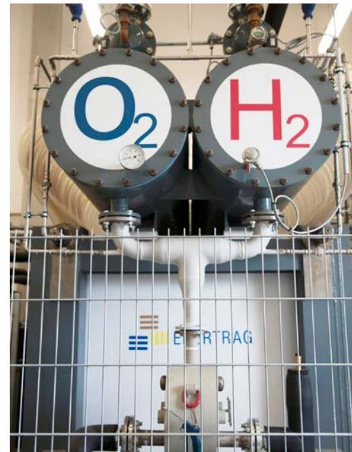
Elektrolyser at the Enertrag hybrid power plant in Prenzlau.
