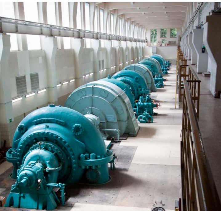
Pumped storage plant in Waldek, Hesse.
