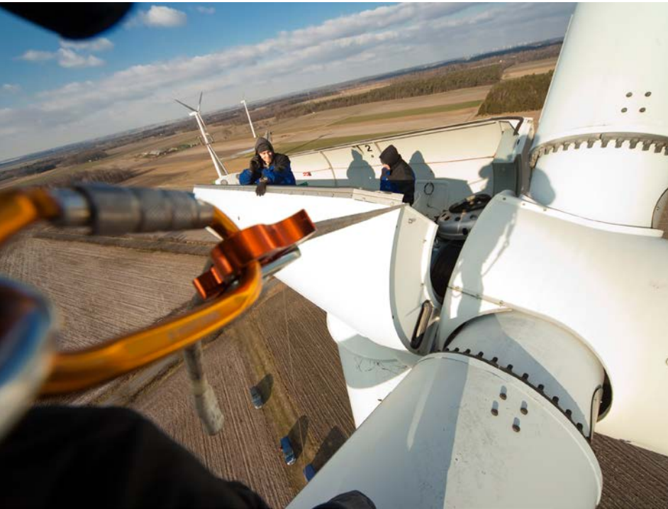
Servicing a Siemens turbine at Uthlede wind farm, Lower Saxony.
